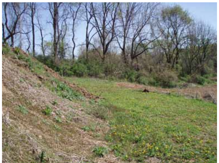
Soil pile and remnants of silt fence
